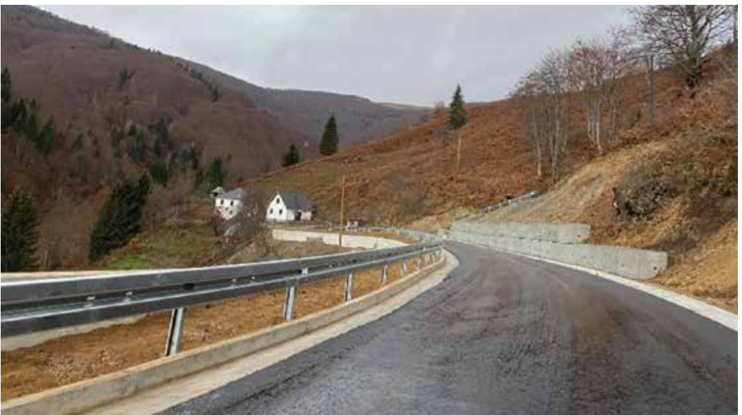
Supervision on the rehabilitation of the landslide "Gnjila Potok" on the road Mateševo–Andrijevića of a landslide approximately 140 m long, within which the reconstruction of the road structure was performed
