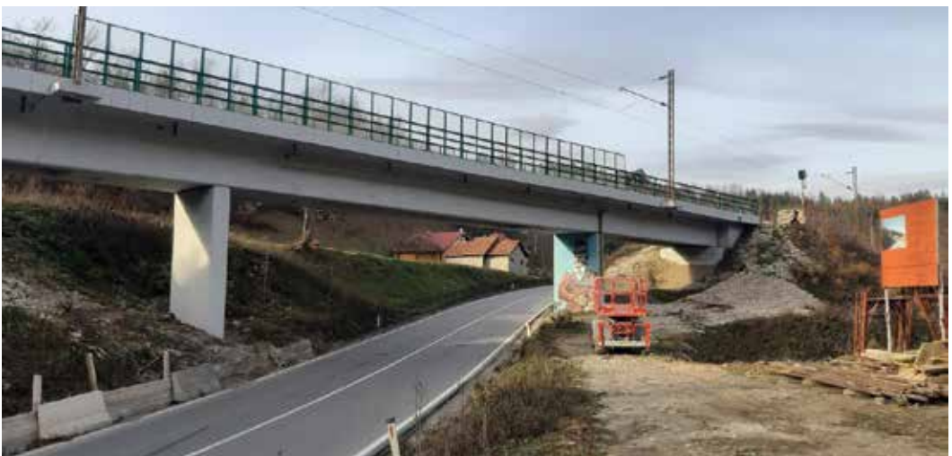
Supervision of the Works on Rehabilitation of 13 concrete bridges on the "Vrbnica-Bar" railway line in Montenegro, Fidic Contract Project
